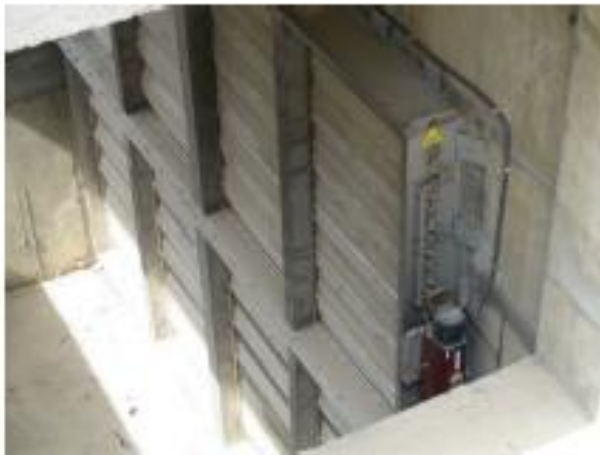
Figure 3 Very poor installation and lack of maintenance on the dampers
