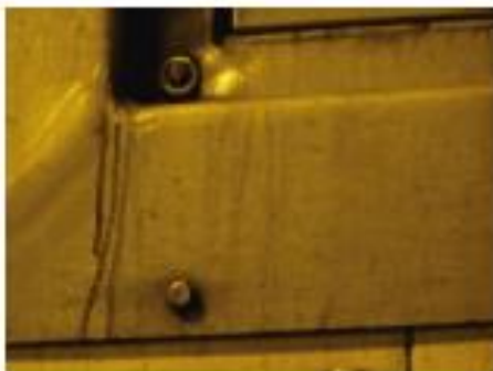
Figure 4 Close-up of the corrosion caused by gap corrosion
