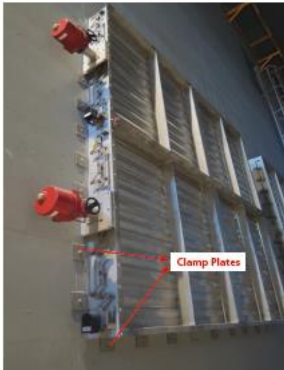
Figure 1 Stainless steel damper installed on to an opening in the wall with clamp plates
