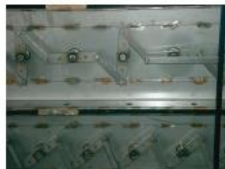
Figure 2 Cross contamination on stitch welds leading to corrosion
